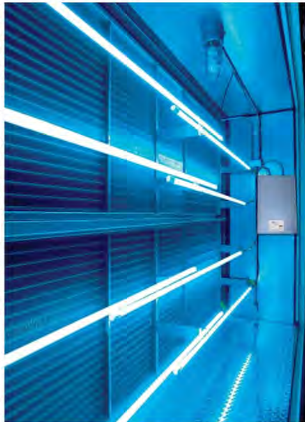
Ongoing crisis has triggered unprecedented interest in UV-C.
